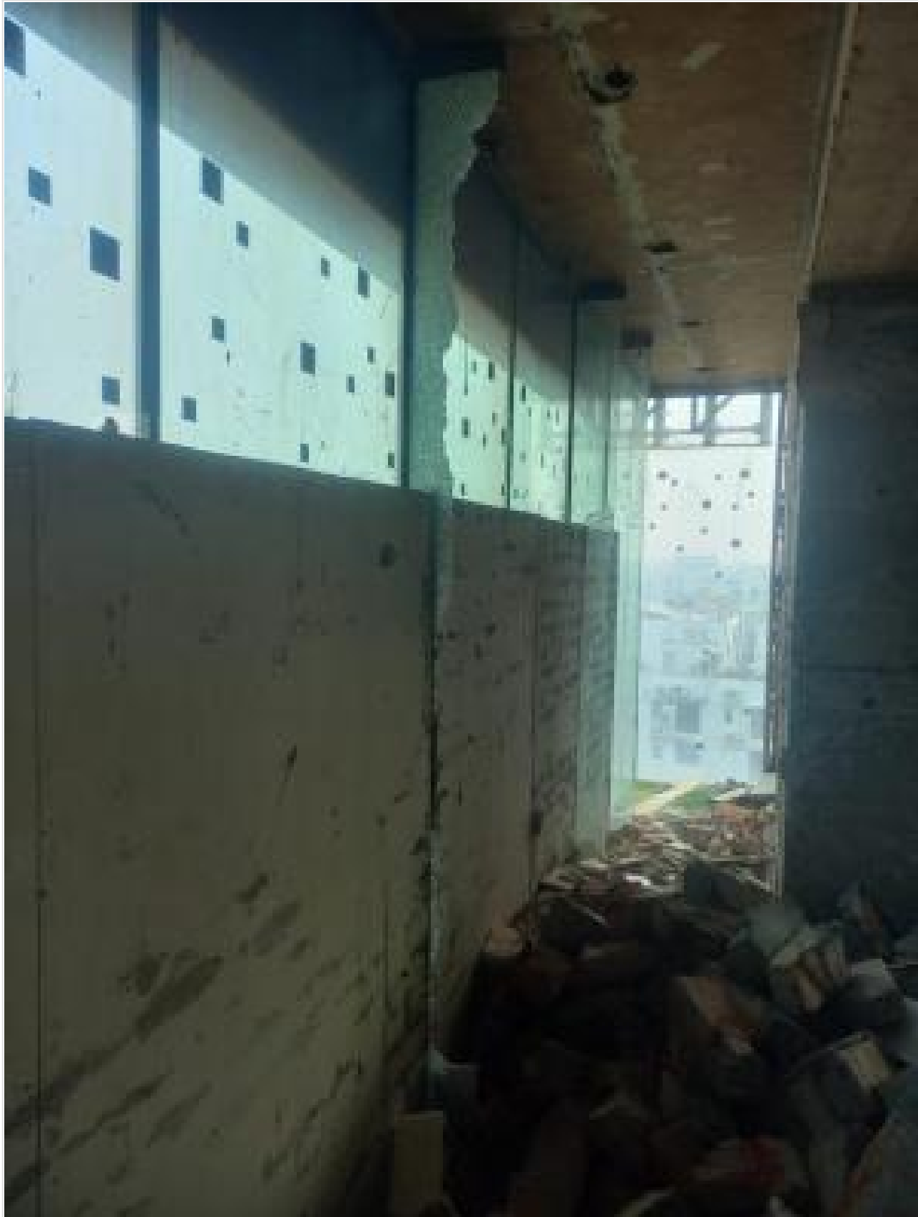
L-14-Fin glass broken during dismantling on 10-10-23
